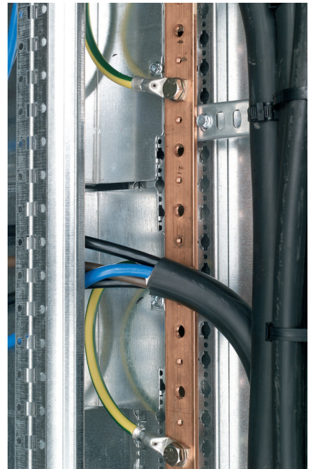
Main terminal in cable sleeve consisting of a 32 x 5 mm copper bar
